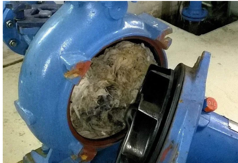
Clogged pump without XRipper
