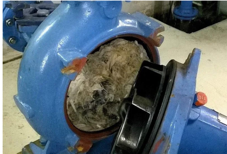
Clogged pump without XRipper
